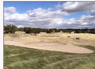
This photo illustrates the construction process for the new tees being added throughout the Sunrise Course. Although this photo is from the Sunset Course, it is a good reflection of the process of identifying tree locations and elevations and the Maintenance Team bringing them to life through rough shaping, drainage installation and sand capping prior to a final final and grassing.
