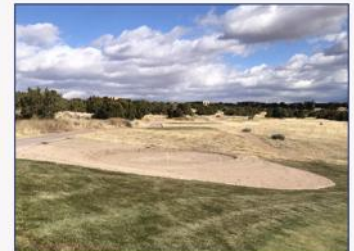
This photo illustrates the construction process for the new tees being added throughout the Sunrise Course. Although this photo is from the Sunset Course, it is a good reflection of the process of identifying tee locations and elevations and the Maintenance Team bringing them to life through rough shaping, drainage installation and sand capping prior to a final float and grading.
