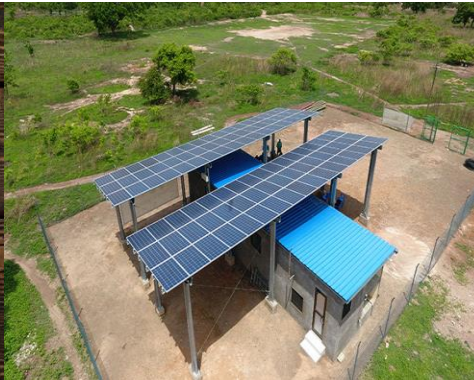
Renewable off-grid Energy
